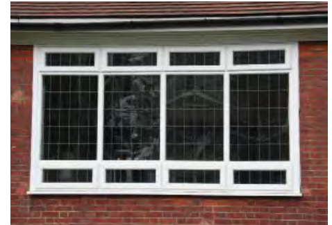
An examples of a replaced window (above bottom) that has significantly departed from its original design (above top)
