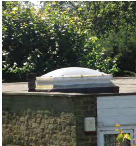
A replaced domed skylight that meets current Building Regulations
