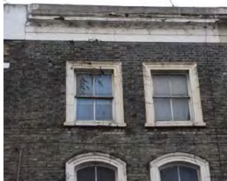
Buildings in a poor state of repair
