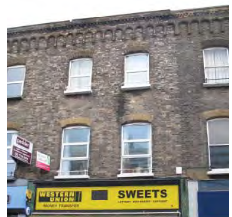
Unauthorised replacement uPVC windows that have had a negative impact on the character of the host building, which would originally have had timber sash windows
