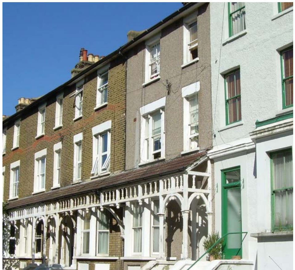
Inappropriate application of pebbledash render to a house in a terrace in the East India Estate Conservation Area has significantly altered its appearance.
