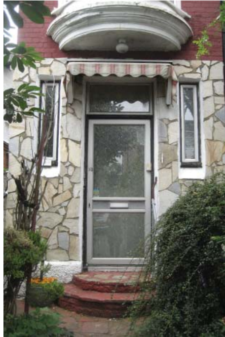
An example of inappropriate installation of an aluminium door. This development has harmed the character and appearance of the conservation area
