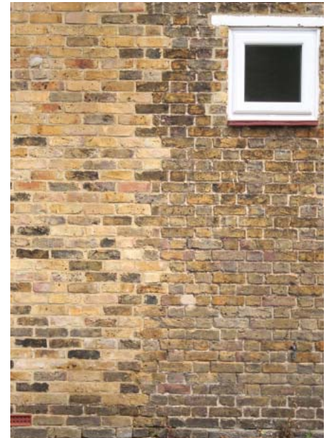
Photograph illustrating a poor matching of bricks for an extension with that of an existing building
