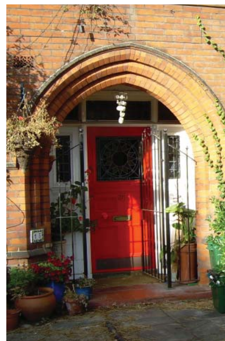
A deep recessed porch with decorative brick moulding and a patterned terracotta string course above
