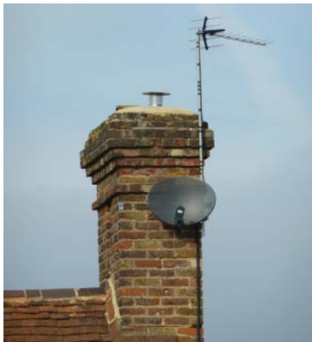
Poor location of equipment
